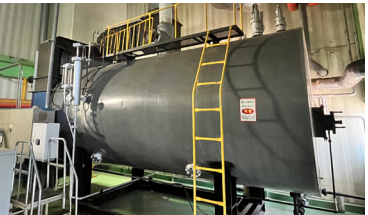
Low-NOx Boiler (10 tons)
