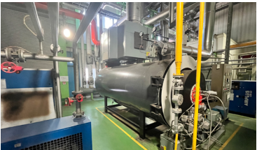
Low-NOx Boiler (3 tons)
